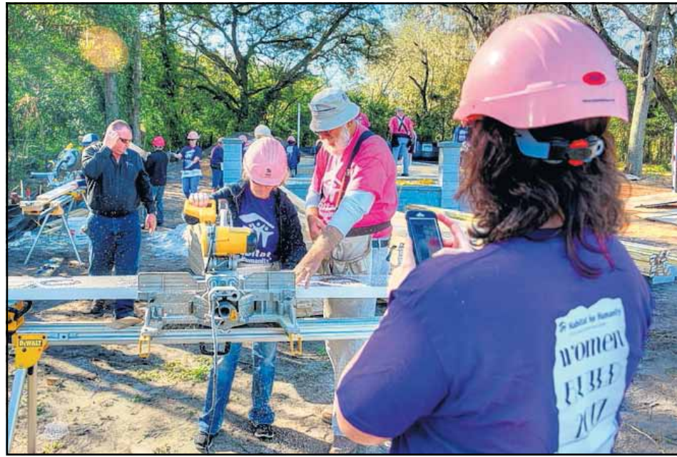
Tera Townsend of Lady Lake, uses a power saw to cut headers for the windows and doors in the home. Earl Cunningham, Habitat Volunteer Supervisor, assists.
