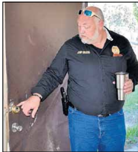
Dade City police Sergeant James Walters points out bullet holes from when officers used a shotgun to breach a door at the empty Dade Oaks apartment complex.
