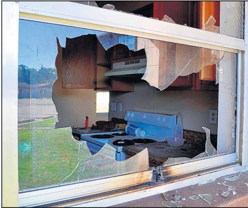
Below the shattered window, a burn mark can be seen from a law enforcement agency that utilized the space to practice with a fire tool for entering buildings.
