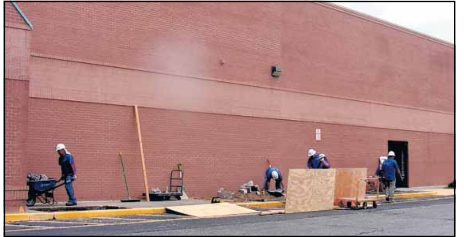
Simpson Environmental Services employees work Tuesday at the future site of the Rural King Supply Store on Gall Boulevard. A July 17 opening is planned.
